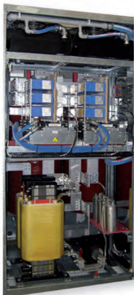
D DC/AC Inverter for energy application, 1200 KVA
