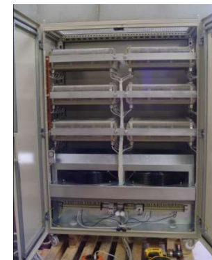
RDP in rack (120KW system)
