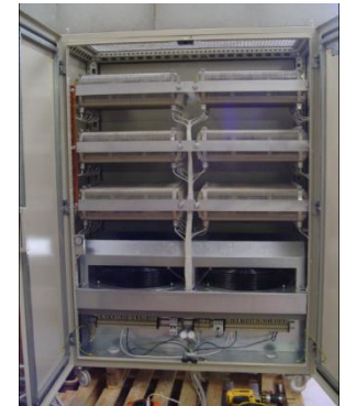
RDP in rack (120KW system)
